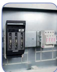
LTL00 disconnector and modular equipment
